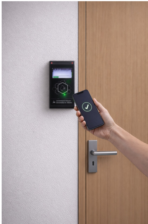
Fig. 1. Installed reader device
