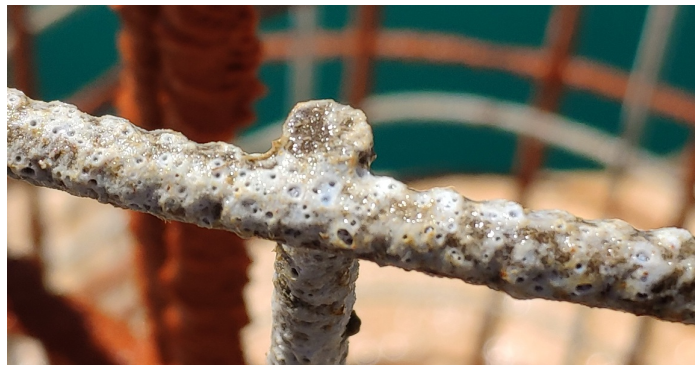
Figure 1: aspect of the calcareous coating at the end of the electrolysis phase.
