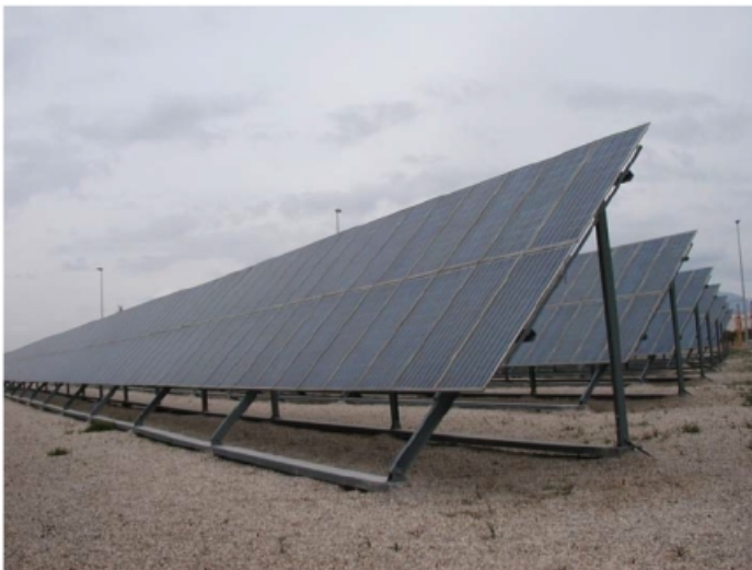
Figure 3. General view of the Photovoltaic Solar Plant of the University of Alicante.
