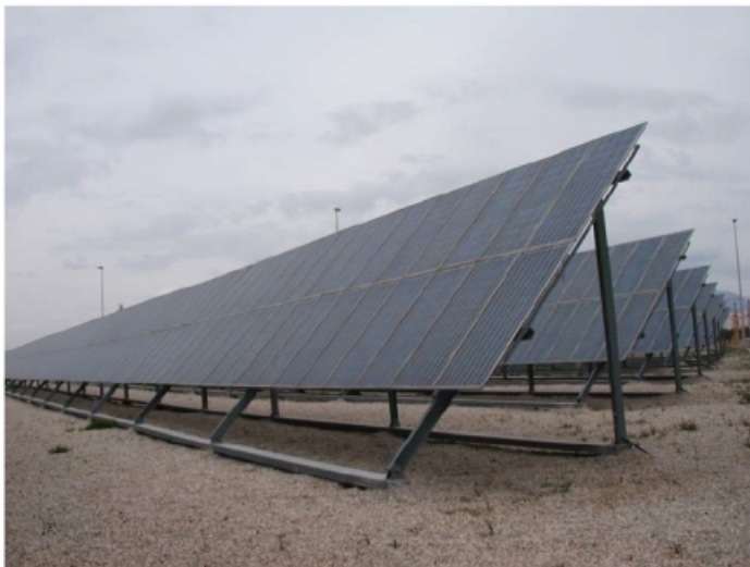
Figure 3. General view of the Photovoltaic Solar Plant of the University of Alicante.
